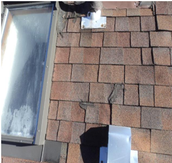
DSC06459.JPG Damaged roof shingles.
