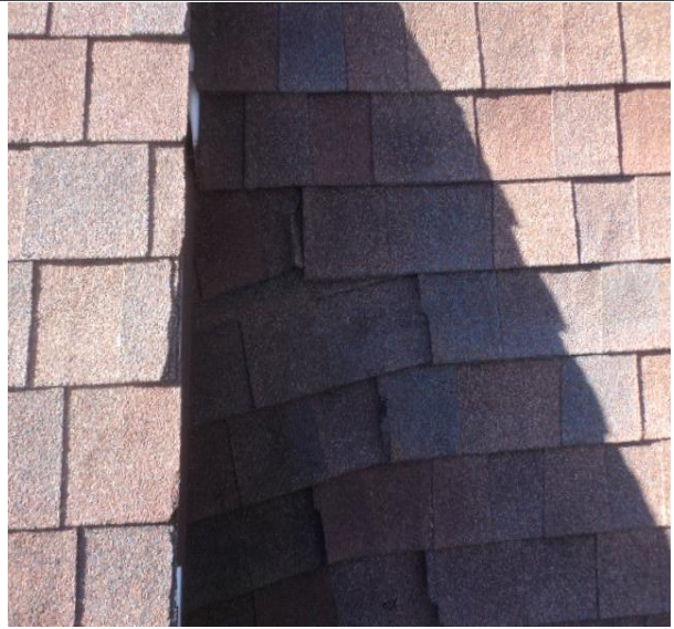
DSC06463.JPG Damaged roof shingles.
