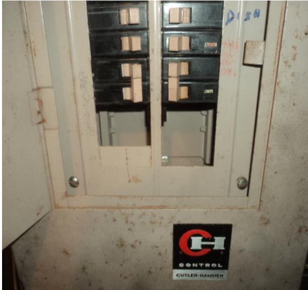
DSC06494.JPG Missing knockout plugs.
