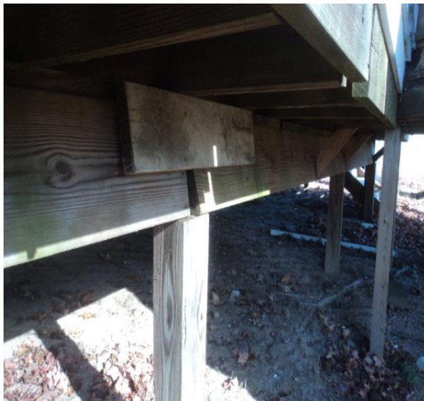
DSC06479.JPG Structural damage to deck stucture.
