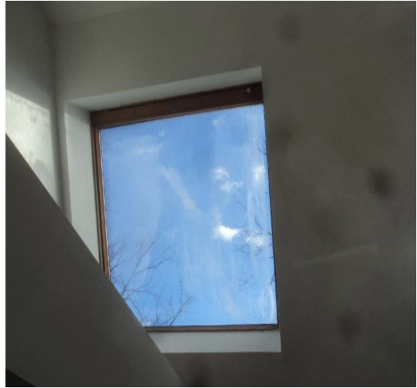
DSC06507.JPG Broken window seal.
