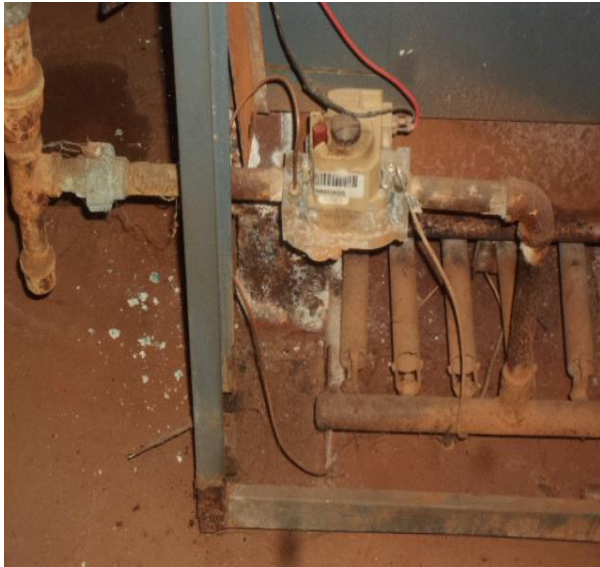
DSC06501.JPG Rusty heat exchanger.
