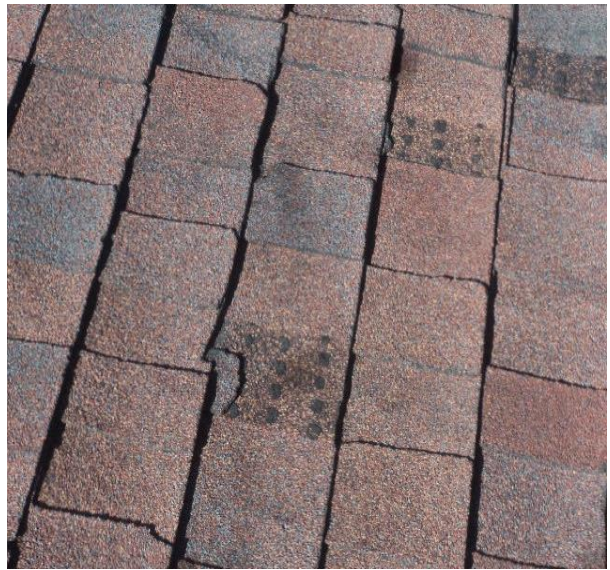
DSC06465.JPG Damaged roof shingles.
