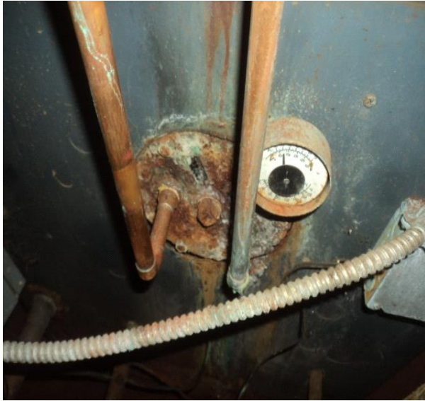
DSC06499.JPG Leaky domestic hot water heat exchanger. Damaged pressure/temperature gauge.
