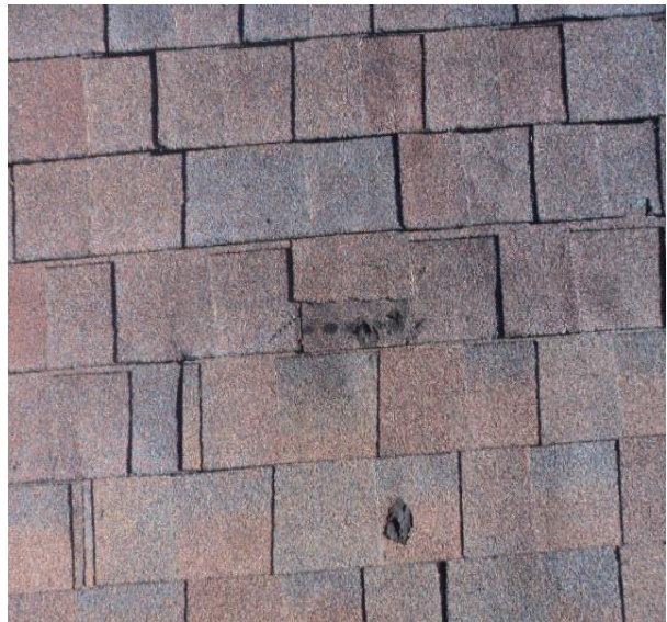
DSC06461.JPG Damaged roof shingles.
