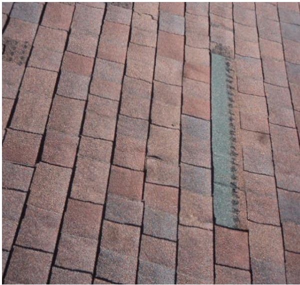
DSC06464.JPG Damaged roof shingles.
