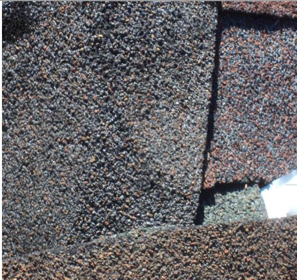
DSC06466.JPG Damaged roof shingles.
