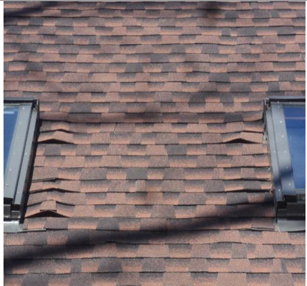
DSC06475.JPG Lifted shingles.
