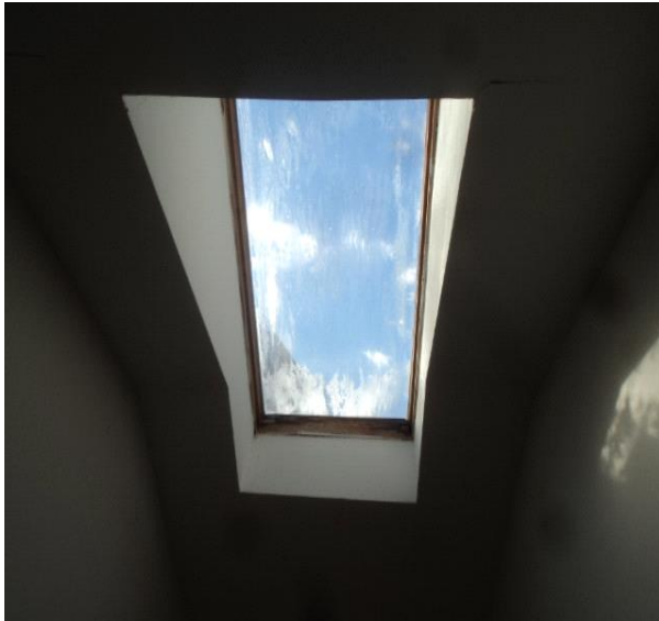
DSC06514.JPG Broken window seal.
