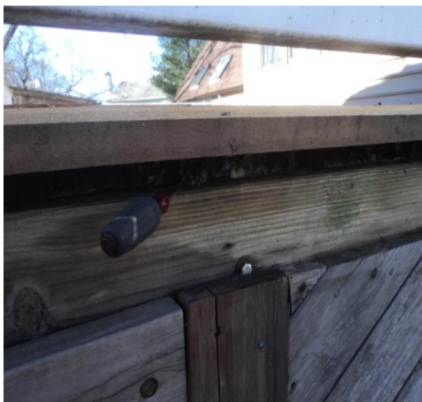
DSC06481.JPG Structural damage to deck stucture.
