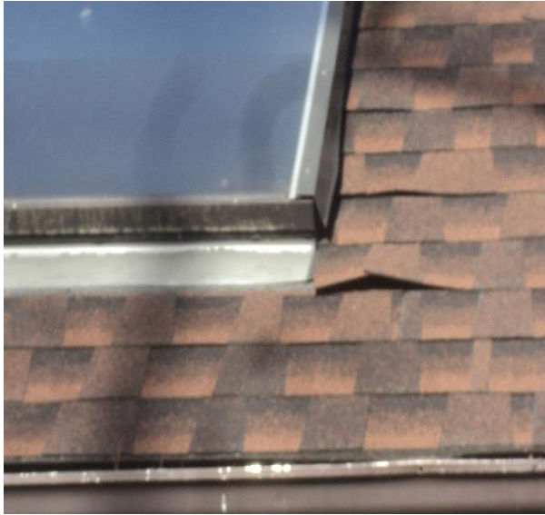
DSC06476.JPG Broken window seal.
