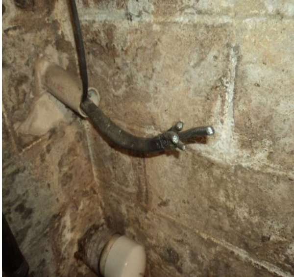
DSC06490.JPG Signs of exterior water penetration into the basement.
