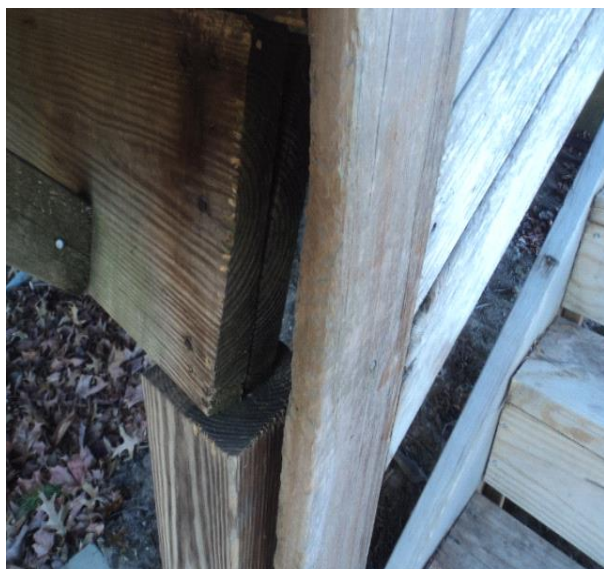
DSC06480.JPG Structural damage to deck stucture.
