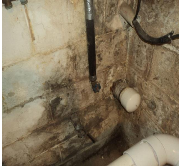
DSC06491.JPG Signs of exterior water penetration into the basement.
