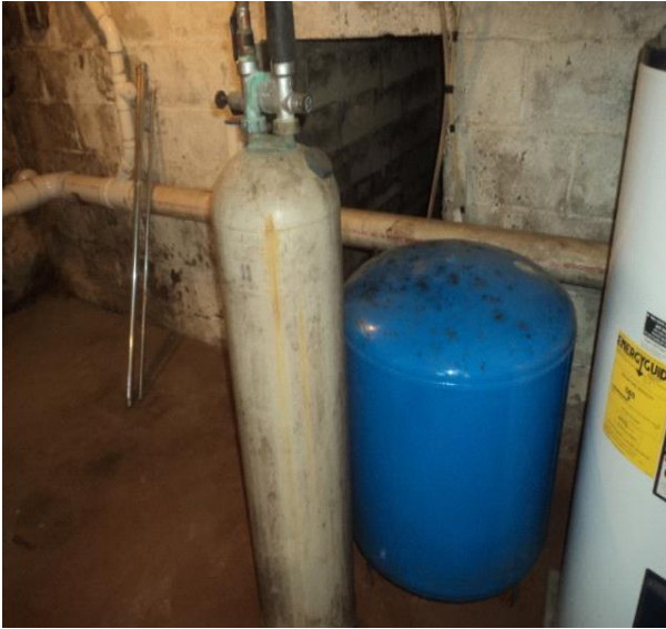
DSC06493.JPG Abandoned private water tank, pump.
