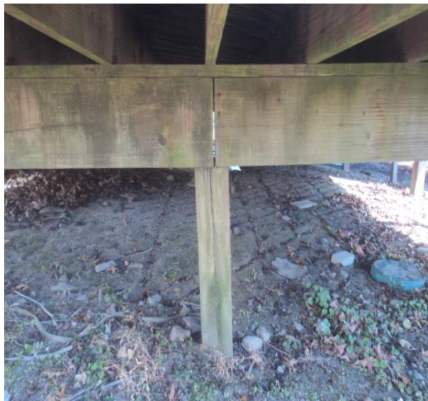
DSC06478.JPG Structural damage to deck stucture.
