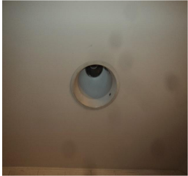
DSC06513.JPG Light fixture in tub area (electrical hazard).
