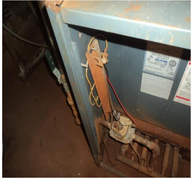
DSC06500.JPG Rusty heat exchanger.
