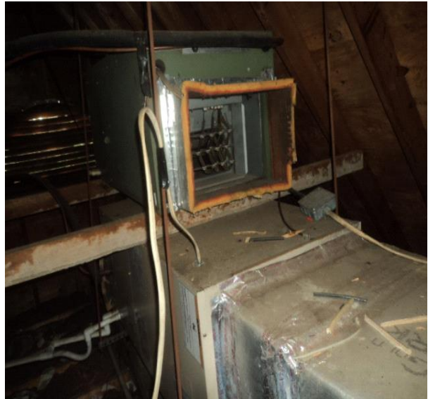
DSC06519.JPG Abandoned old A/C interior unit in the attic.
