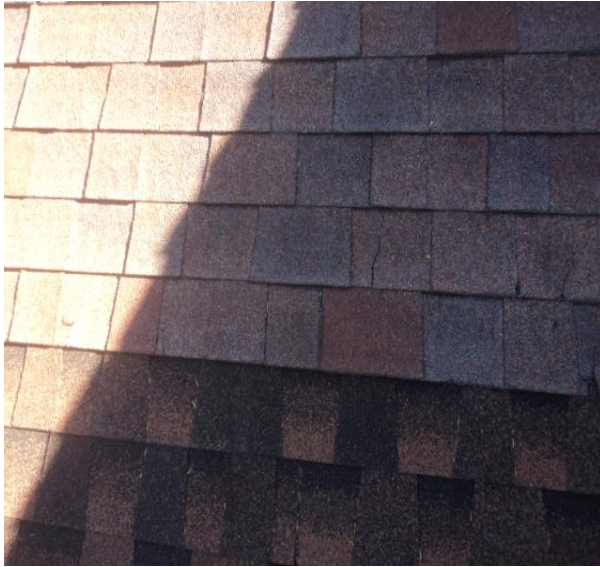
DSC06457.JPG Damaged roof shingles.
