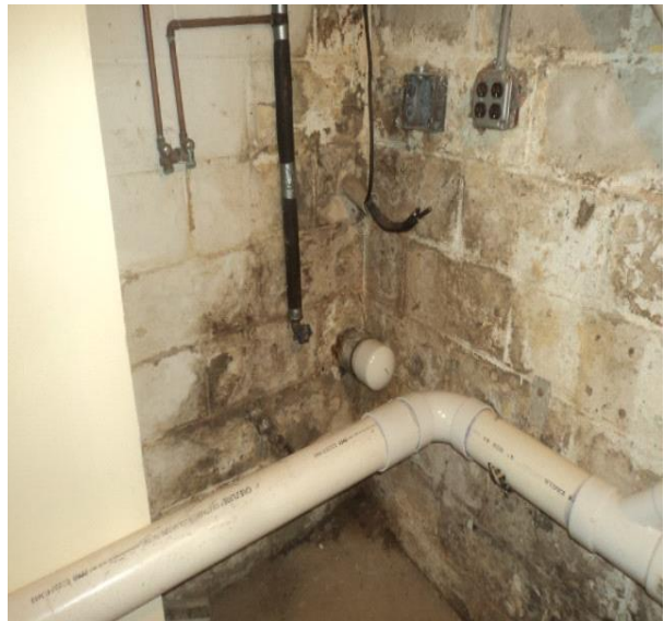
DSC06489.JPG Signs of exterior water penetration into the basement.
